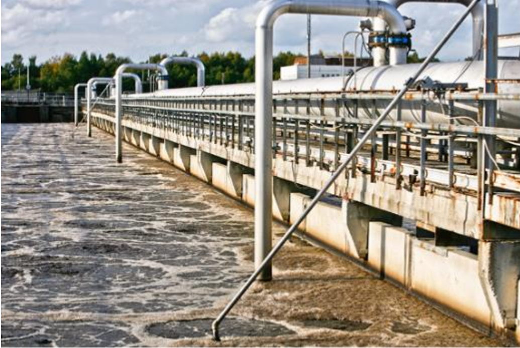
Figure 1.3. Wastewater treatment at Daugavgrīva WWTP (photo F64).
